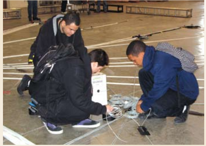
The Big Leagues. Pictured here are some of the 80 technicians from Smart City who wired the exhibit floor. Staff members consider it a point of professional pride to say they worked the CES.
